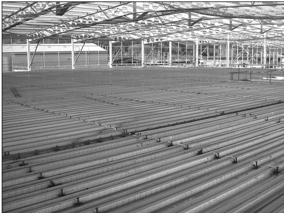
Figure 1.1 A typical example of composite floor construction, showing decking placed on a steel frame
